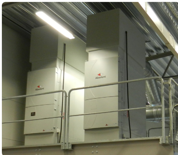
2 A•smoke 80TF units with joint A•monitor
